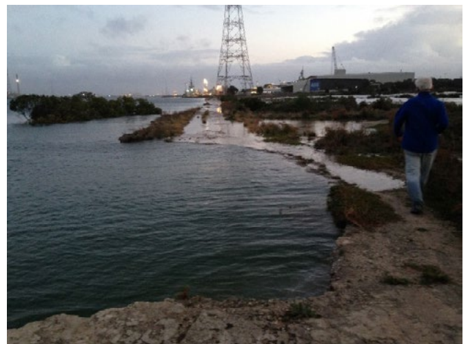
Figure 8: May 2016 storm breaking Mutton Cove levee bank. © Jean Turner.
